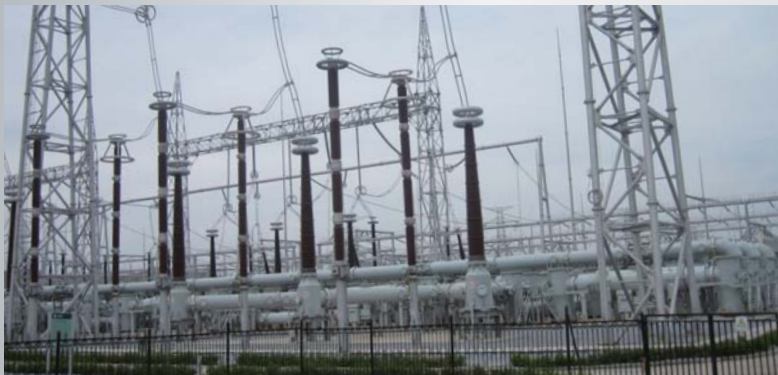
GIS type ZF15-800 in operation at Xining 750kV S/S
