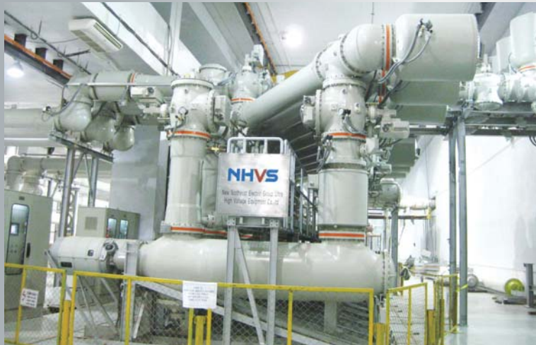
ZF15-550kV GIS in Sonla Hydropower Substation in Vietnam
