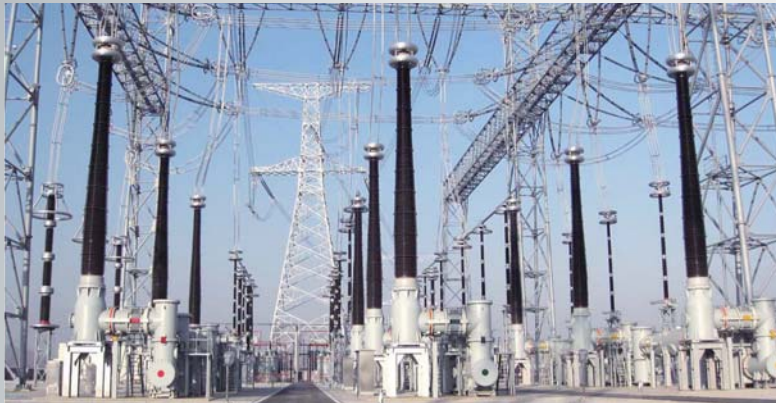
NHVS 1100kV HGIS in Nanyang Substation
